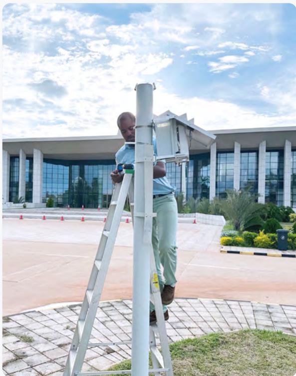
Technician installs an air quality monitor in The Gambia, expanding a nationwide network that tracks pollution in real time.
